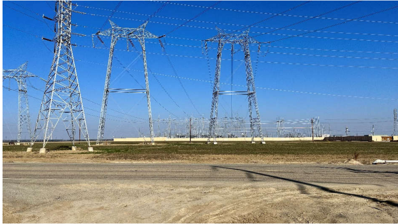
Photograph 13. View of the northern adjacent PG&E substation, facing north across West Jayne Avenue.
