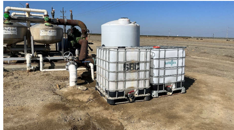
Photograph 6. View of the tote tanks, sulfuric acid AST, and associated irrigation equipment observed along the northern boundary of the subject property.
