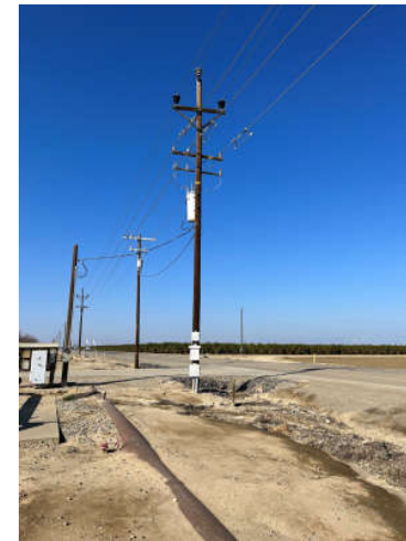
Photograph 4. View of a pole-mounted transformer on the northwestern corner of the subject property.
