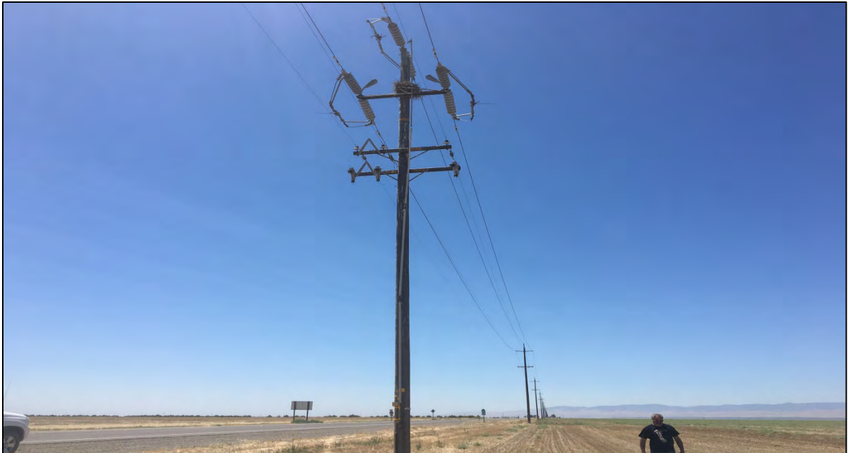
Photo K: Close-up view of large stick nest on top of a utility pole, outside the eastern project limits, in the SR-33 right-of-way, approximately 435 feet south of West California Avenue (June 20, 2016).
