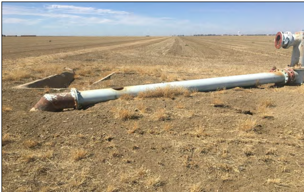
View of abandoned water pump and pipe, and California ground squirrel burrows that provide suitable habitat for burrowing owls, located 20 feet north of West Jensen Avenue 0.50 mile east of South Ohio Avenue, looking north (June 20, 2016).
