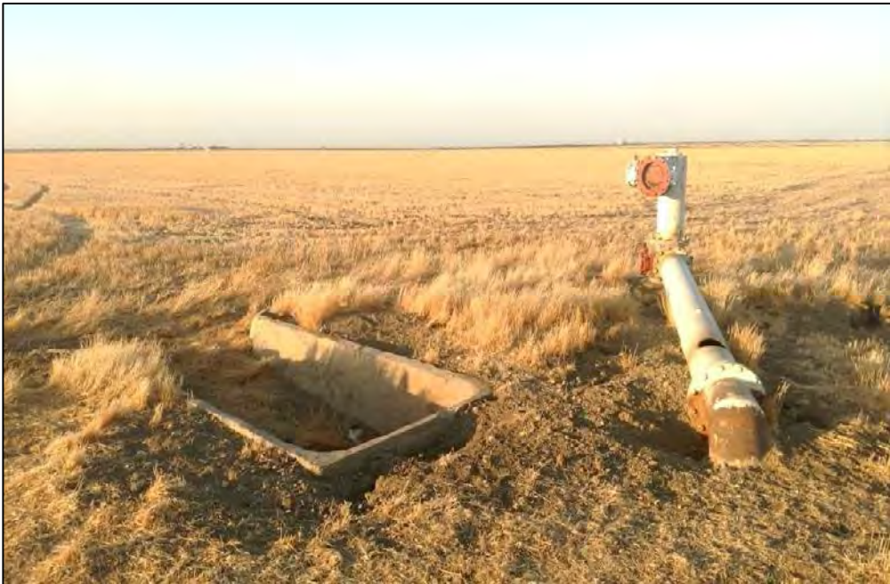
Photo 7f: View northeast at concrete culvert and abandoned water pump pipe just north of West Jensen Avenue and just east of Ohio Avenue. No burrowing owls or sign of the presence of burrowing owls were observed at this location (July 12, 2017).
