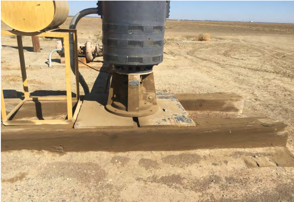
Site 7: Ag pump and turbine oil AST. Soil staining present around all sides of pump base.
