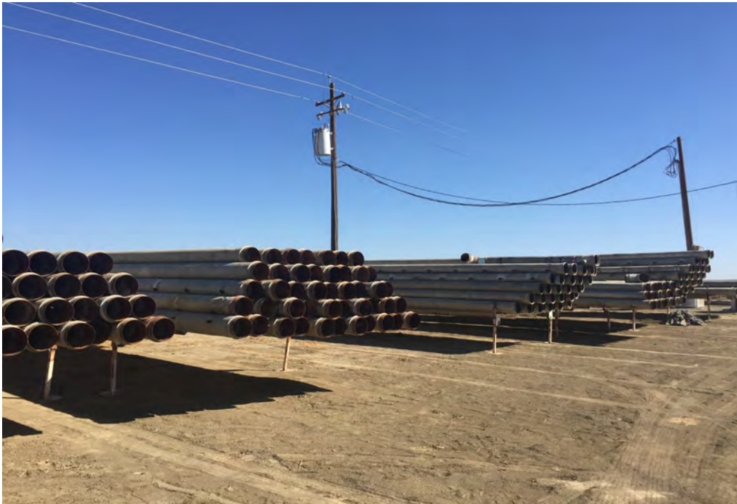
Site 7: Pipe laydown area and pole mounted transformer.
