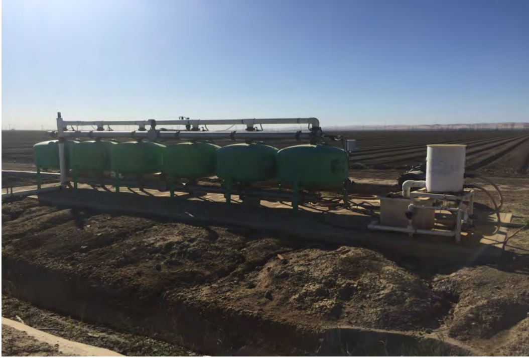
Example of a water filtration system located across the site.
