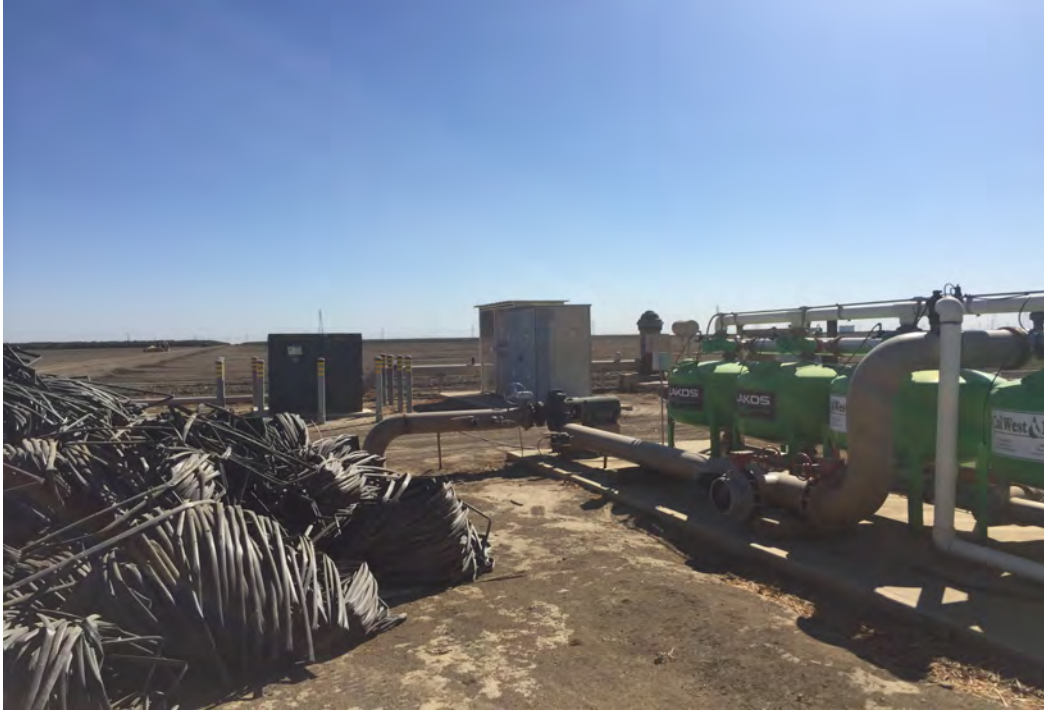
Site 8: Filtration system, ag pump with turbine oil AST with soil staining around base of pump, pad mounted transformer, electrical panel, two square poly tanks containing corrosive liquid.
