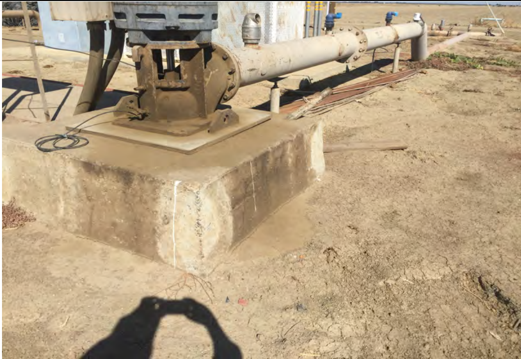
Site 8: Concrete and soil staining around base of pump.
