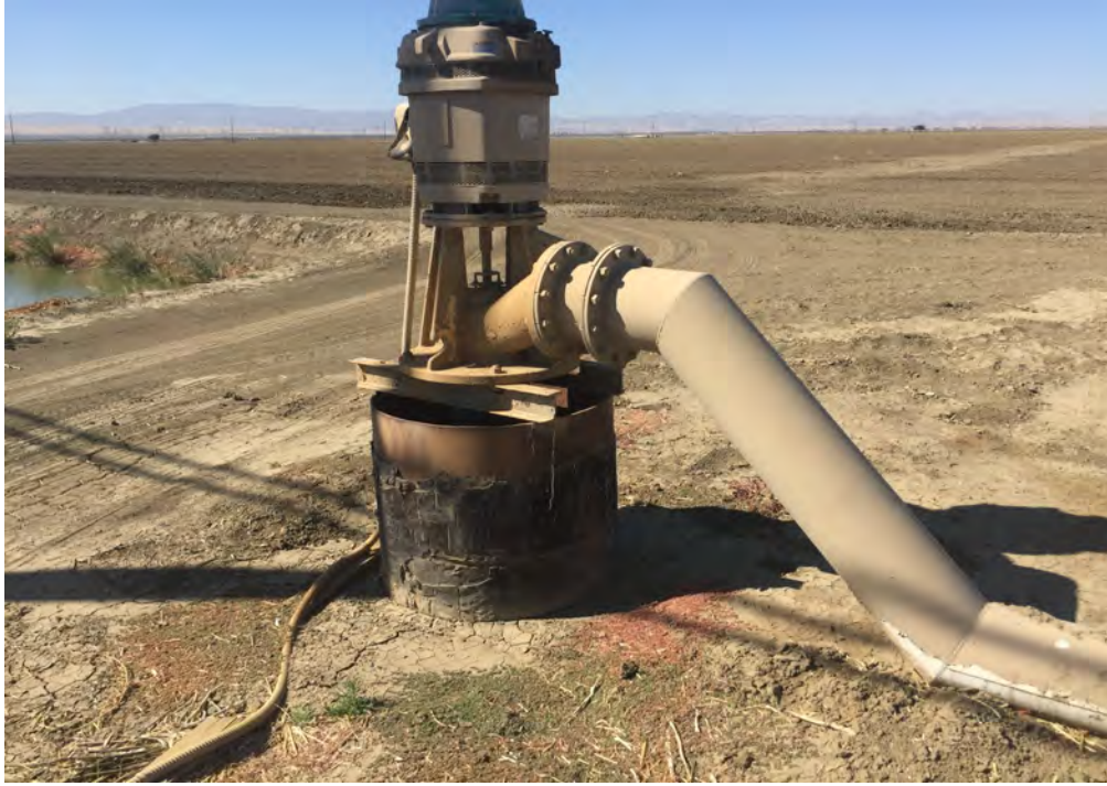
Water pump located along Lassen Avenue. No staining on or below pump.
