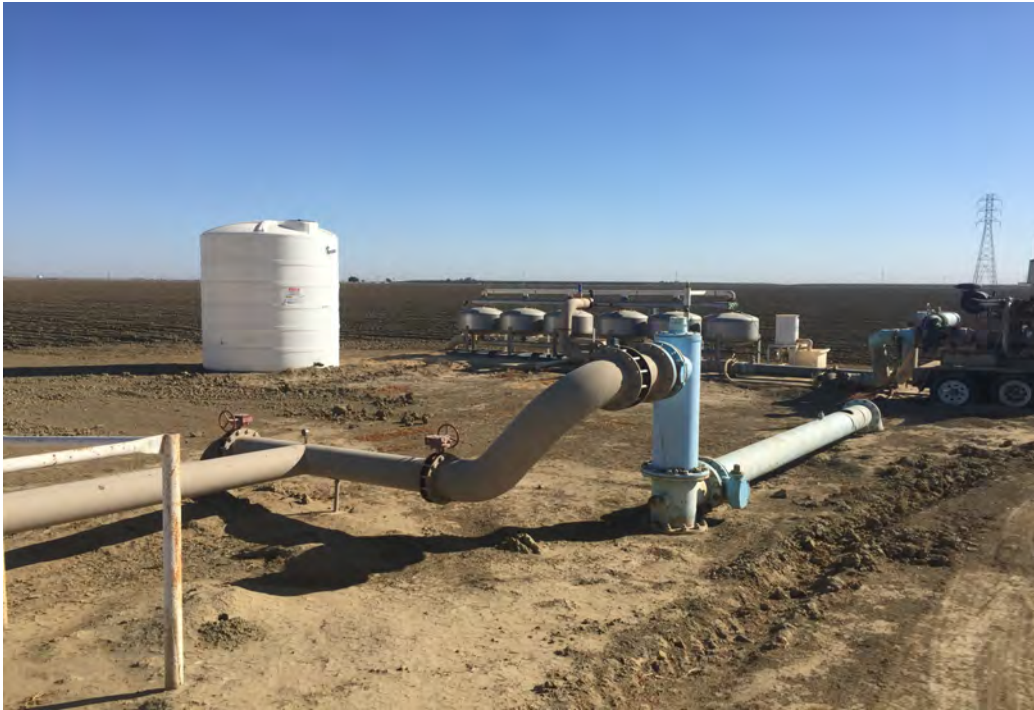
Site 5: Large white poly tank, filtration system, trailer mounted diesel ag pump (with staining) and Westlands Water Valve.
