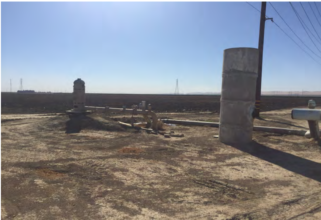
Site 4: Concrete standpipe, Westlands Water Valve, pole mounted transformer and ag pump with soil staining at base of pump.
