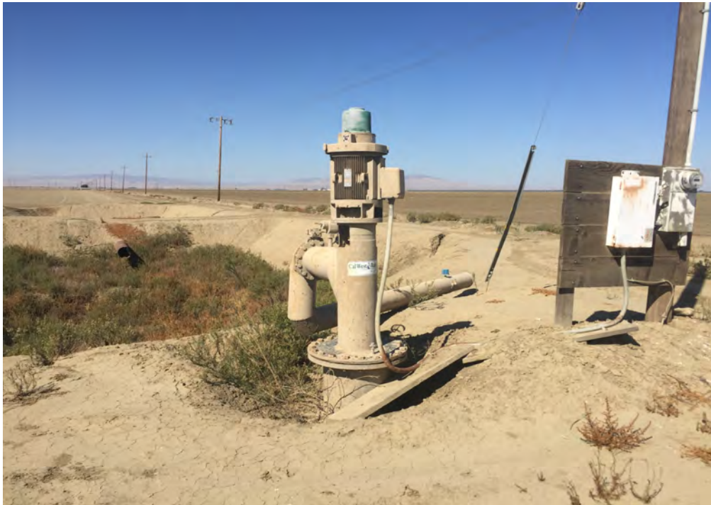
Water pump associated with dual retention basin located along Lassen Avenue. No staining on or below pump.
