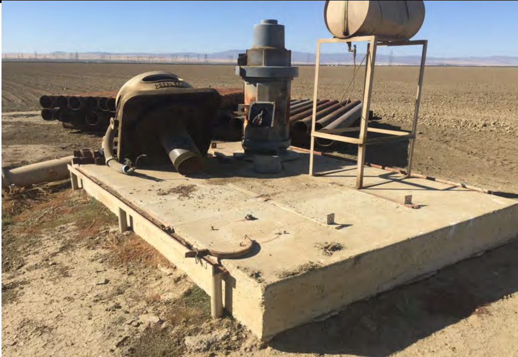
Site 6: Concrete pad, turbine oil AST, ag pump disassembled and inactive ag well. See site notes.
