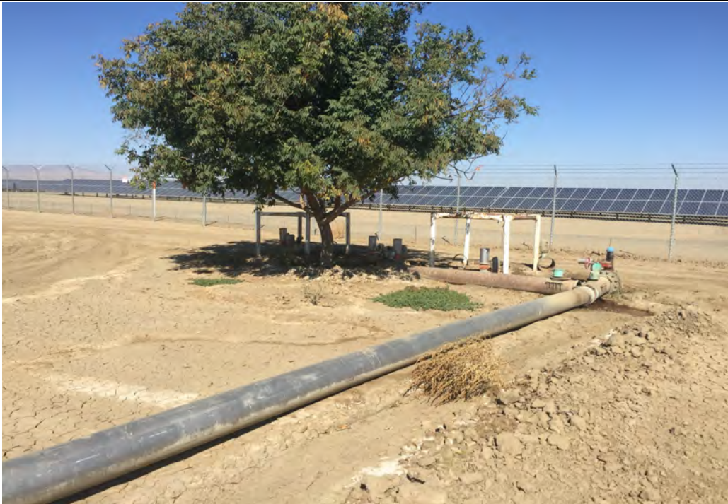
Example of roadside water valves located throughout the site.
