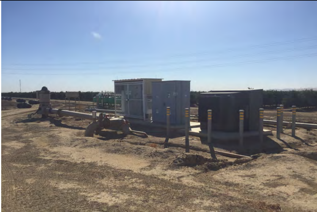
Site 3: • Diesel ag pump on trailer with soil staining under trailer, ag pump with turbine oil AST and staining around of pump, pad mounted transformer, electrical panel, filtration system. See site notes.
