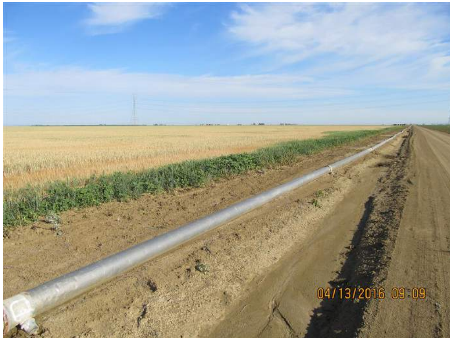
Photo 4. Temporary ditch and a wheat field typical of the southwest quadrant of the site.
