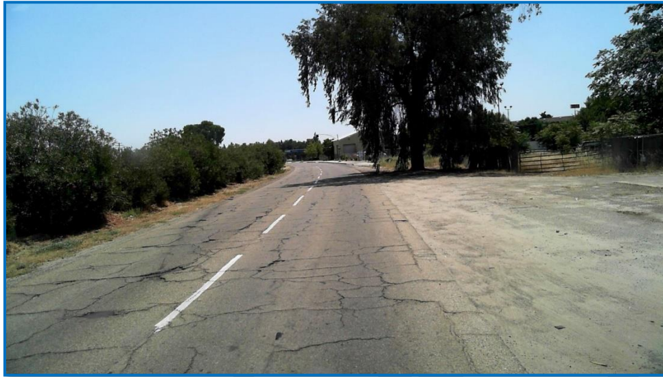
Figure 29 - SB at Sta. 412+80 Representative Pavement Condition
