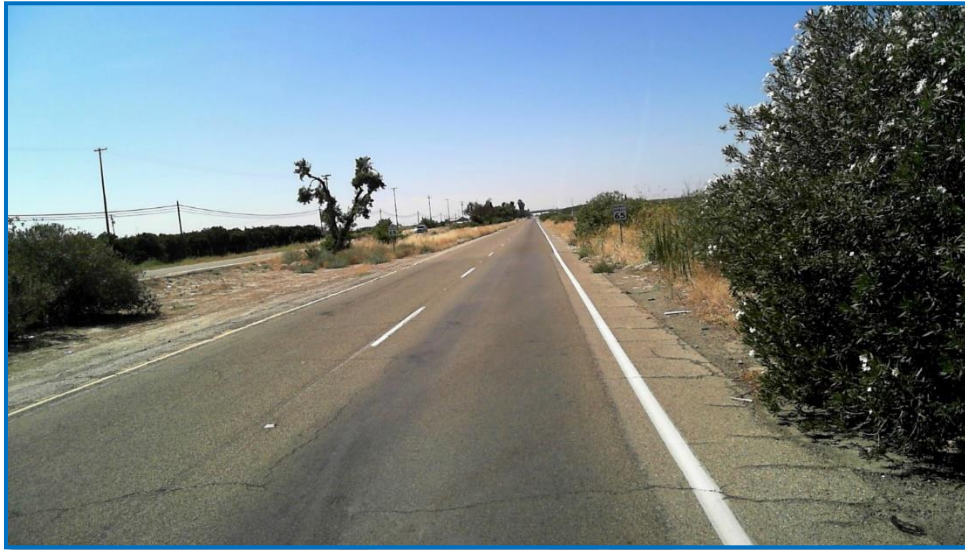
Figure 5 - NB at Sta. 124+44 Representative Pavement Condition
