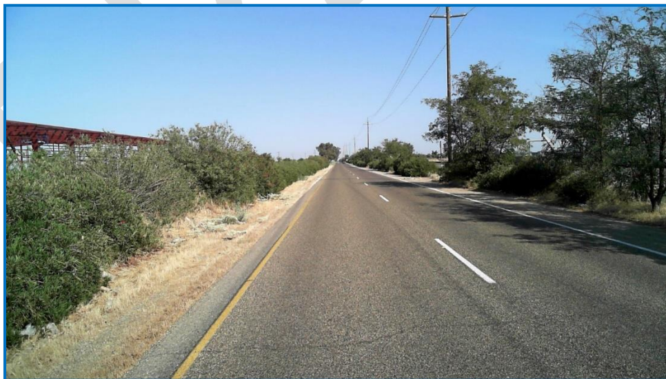
Figure 18 – NB at Sta. 593+70 Representative Pavement Condition
