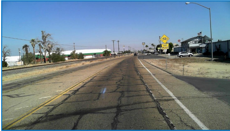
Figure 35 - SB at Sta. 691+05 Representative Pavement Condition
