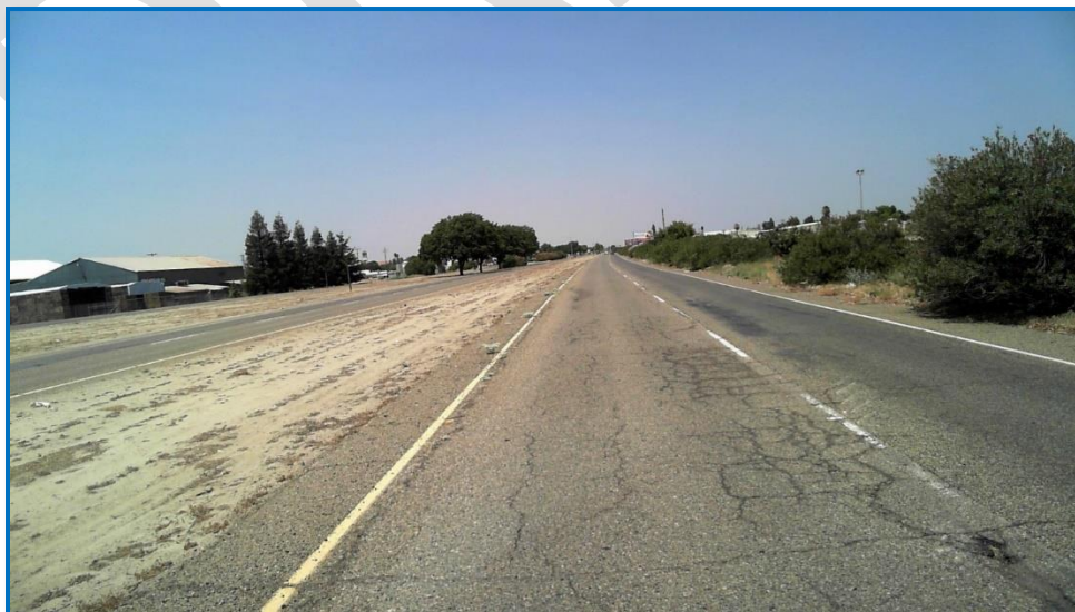
Figure 10 – NB at Sta. 202+20 Representative Pavement Condition
