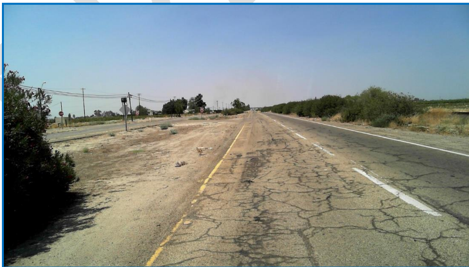
Figure 6 - NB at Sta. 133+95 Representative Pavement Condition
