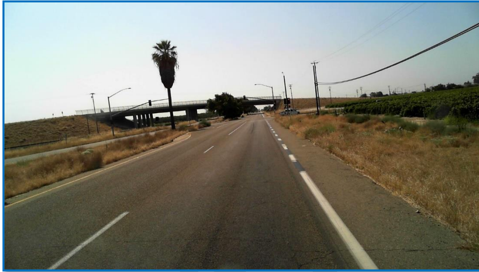
Figure 21 - SB at Sta. 74+55 Representative Pavement Condition
