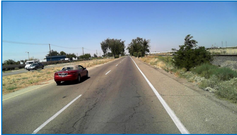
Figure 13 – NB at Sta. 353+94 Representative Pavement Condition
