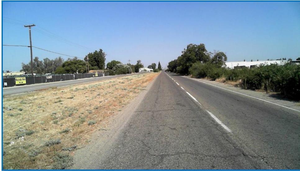
Figure 17 – NB at Sta. 520+20 Representative Pavement Condition
