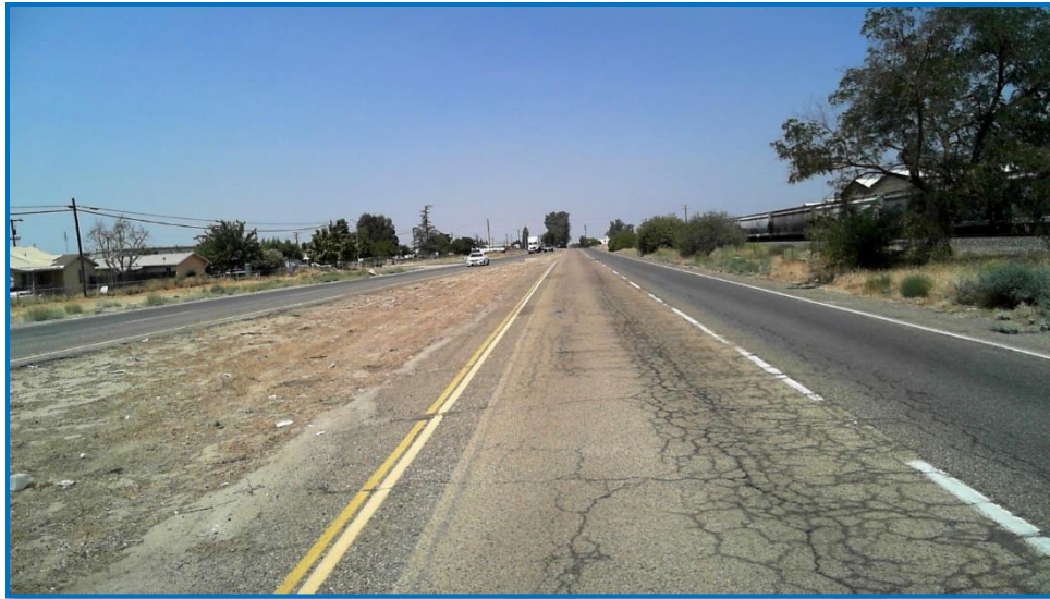
Figure 11 - NB at Sta. 259+20 Representative Pavement Condition
