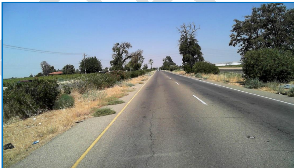
Figure 12 - NB at Sta. 341+45 Representative Pavement Condition
