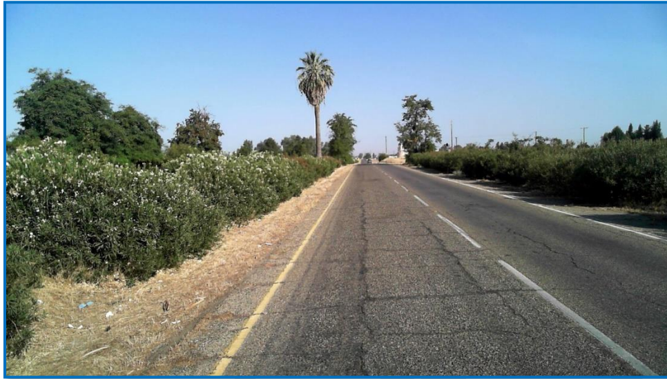
Figure 19 - NB at Sta. 659+45 Representative Pavement Condition
