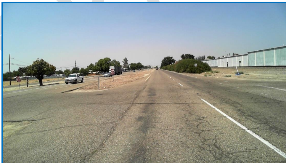
Figure 8 - NB at Sta. 158+20 Representative Pavement Condition
