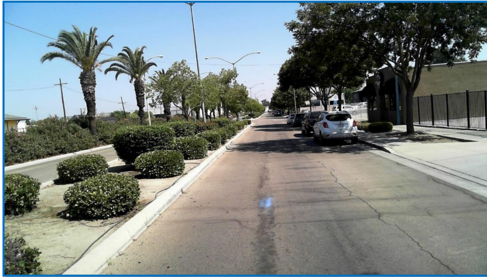
Figure 37 - SB at Sta. 735+80 Representative Pavement Condition
