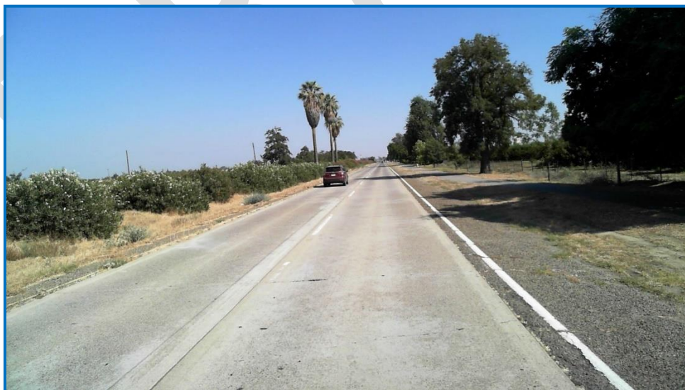
Figure 34 - SB at Sta. 657+30 Representative Pavement Condition
