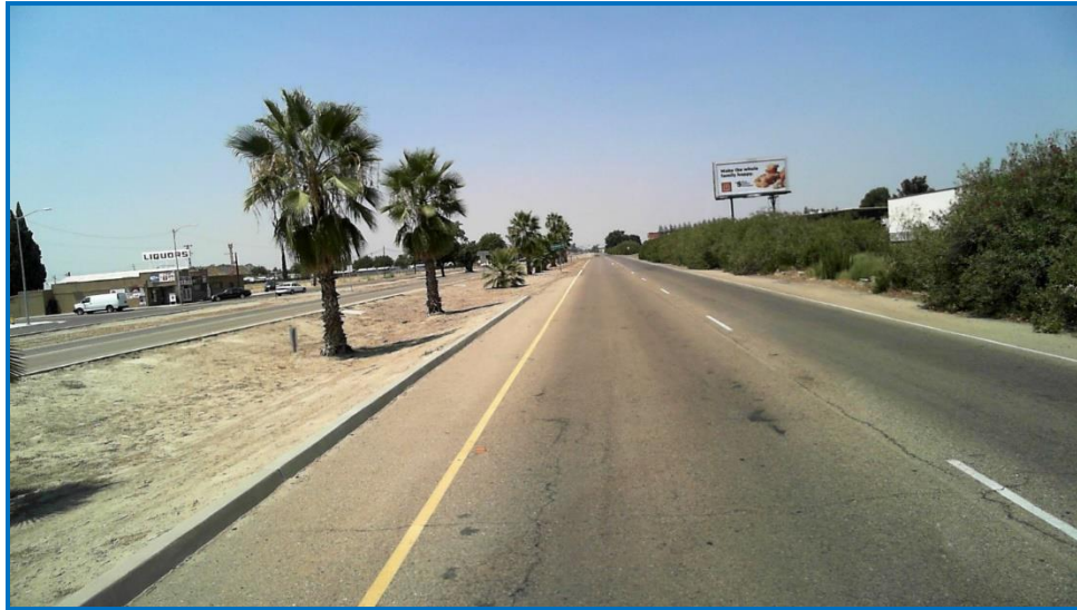
Figure 9 – NB at Sta. 165+20 Representative Pavement Condition
