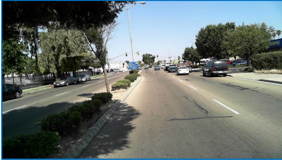
Figure 15 - NB at Sta. 477+45 Representative Pavement Condition
